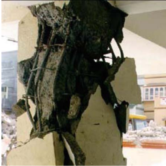
Fig. 6.2 Shear failure of column (See also Plate 5 in Color Plate Section on page 457)
