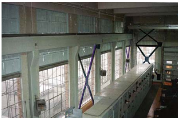
Fig. 6.13 Friction dampers in Pump House Building
