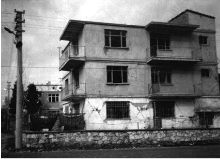
Fig. 8.2 Poor material and mortar in the ground floor (the other two stories are added later)
