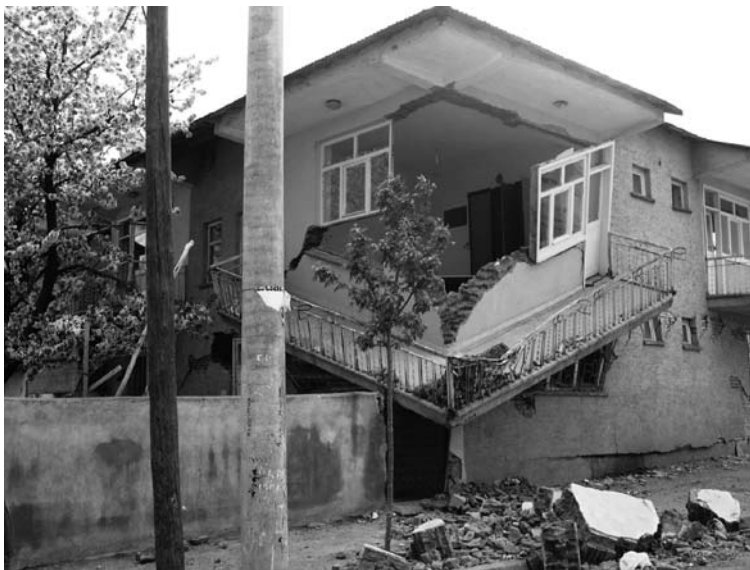
Fig. 8.11 Lack of integrity between walls
