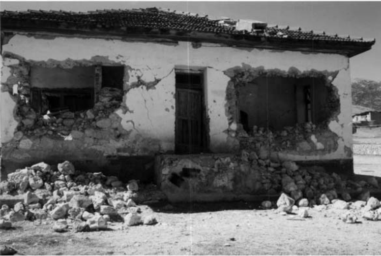
Fig. 8.9 Substandard wall units
