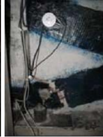
Rupturing of CFRP
