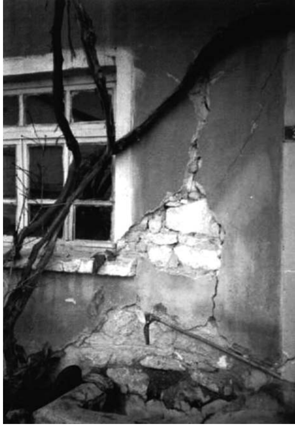
Fig. 8.1 Poor material and mortar in the wall
