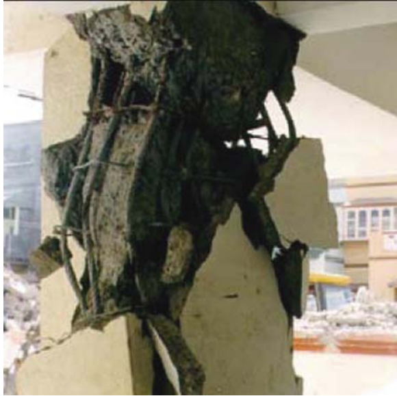
Plate 5 Shear failure of column (see also Fig. 6.2 on page 114)
