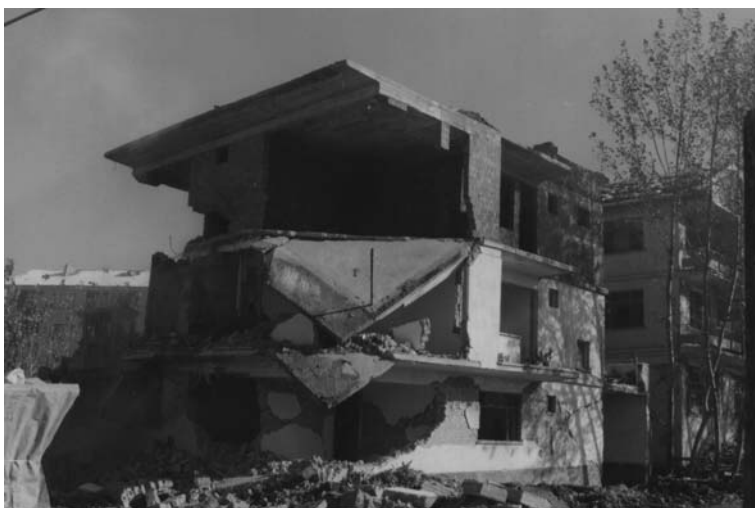
Fig. 8.5 Substandard wall units
