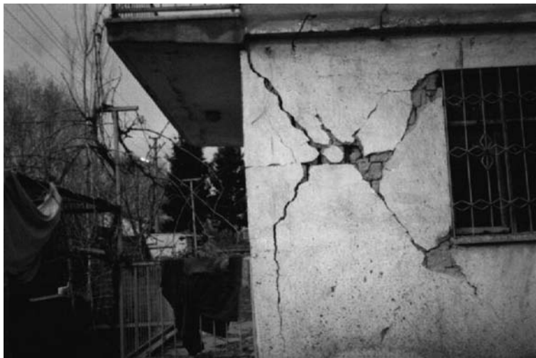
Fig. 8.4 Poor material and mortar in the wall
