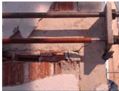
Shear cracks at beam-column joints
