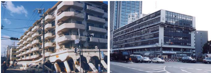
Plate 14 Damages of soft-first-story buildings during Kobe earthquake (see also Fig. 11.1 on page 212)
