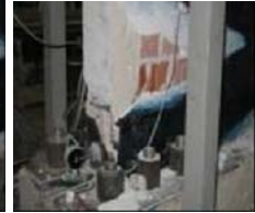
Crushing of cover concrete
