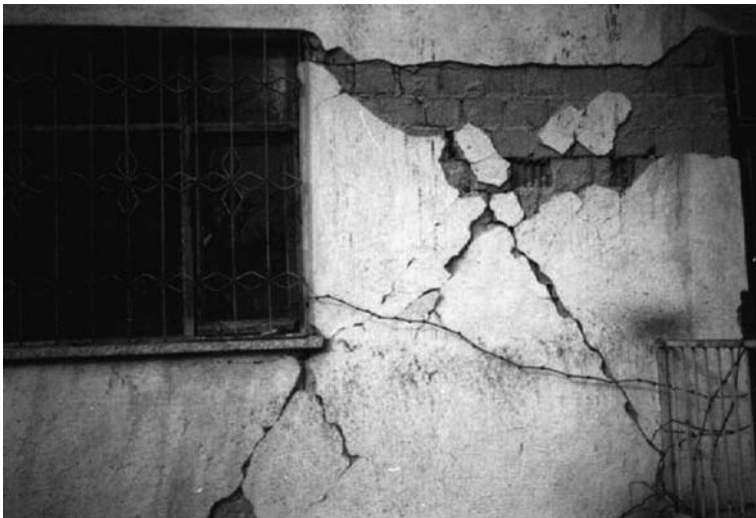
Fig. 8.3 Poor material and mortar in the wall
