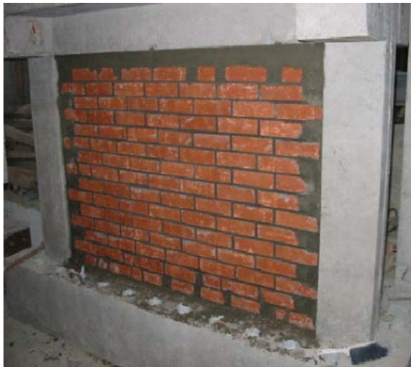
Fig. 19.16 Strengthening of a bare frame by integrated high strength bricks (See also Plate 35 in Color Plate Section on page 474)
