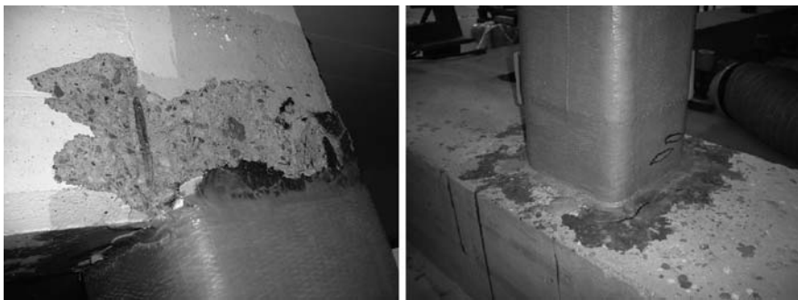
Fig. 5.8 Post-test visual inspection and damage detection after the tests in the FRP-retrofitted configuration
