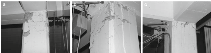
Fig. 5.4 Damaged structure after 0.2 g PGA test: (a) C3 at 2nd storey; (b) C3 at 2nd storey; (c) C4 at 2nd storey
