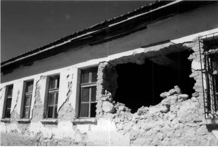
Fig. 8.8 Substandard wall units
