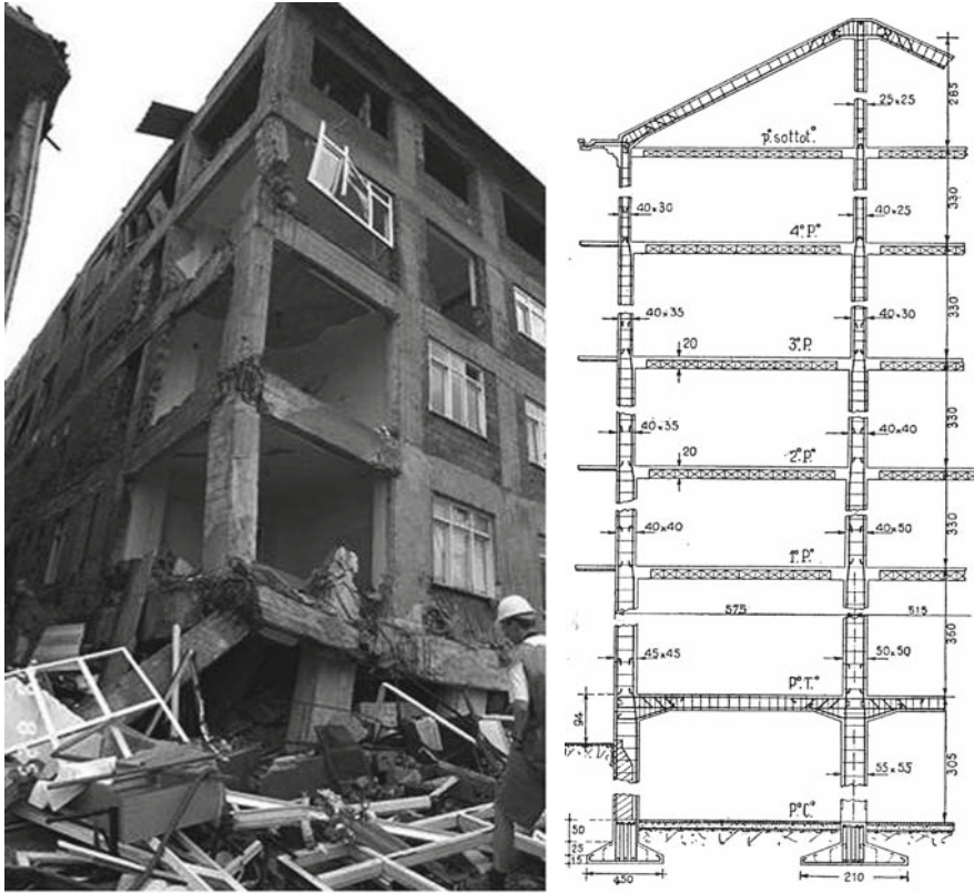
Fig. 13.2 Left : observed damage in a pre-1970s existing reinforced concrete frame buildings with masonry infills (Izmit-Kocaeli earthquake, 1999, courtesy of EERC Library, Berkeley, NISEE Image Collection). Right : typical section elevation of a RC frame building designed in Italy in the late 1950s (after [22])
